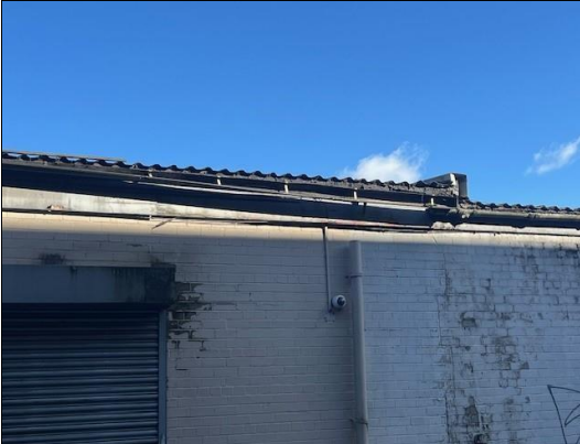
Photo 9 Location: Rainwater goods
