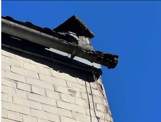
Photo 10 Location: Rainwater goods
